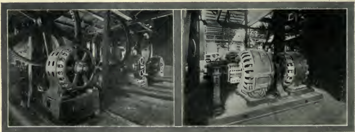
ALDRICH PUMP MOTORS.
